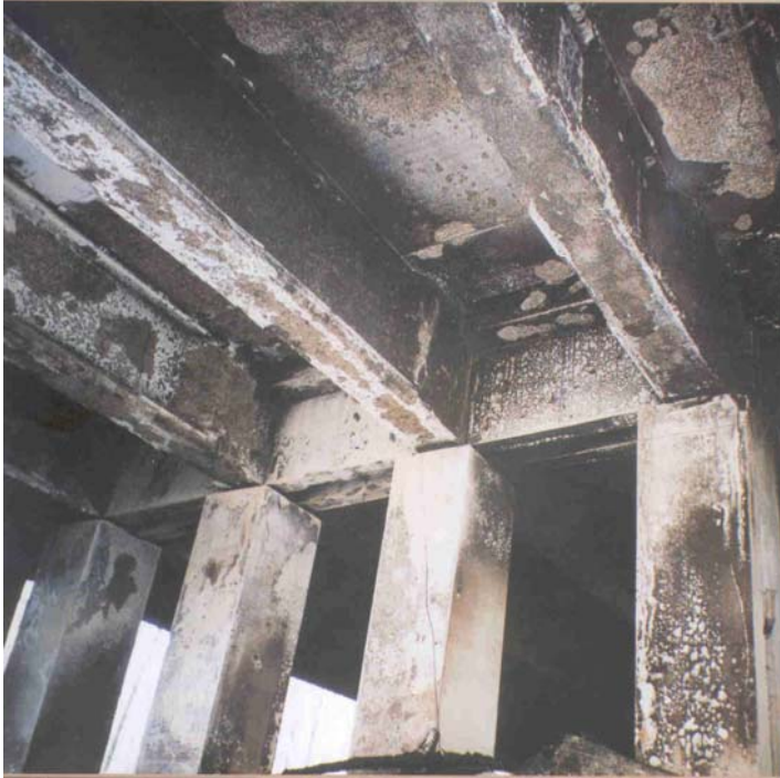
Beneath the bridge deck after the fire (source: ANPI).
