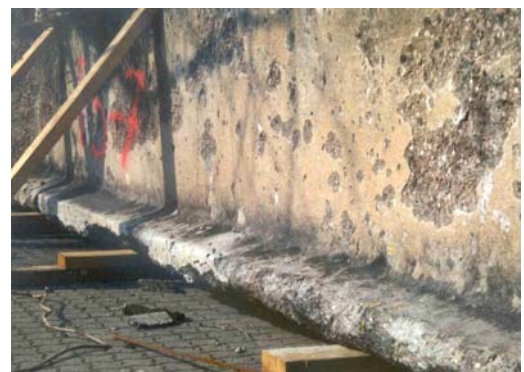
Spalling of the concrete on the main girders (source: FEBELCEM).
