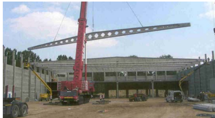
Honda – Alost [58]: (source ERGON) The 50 metre mark is passed. Compartmentalisation is by girders, without openings.
