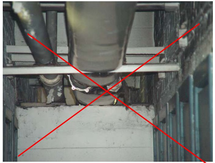
Non re-faced wall in an EI wall, at the level of the heating ducts crossing it (source [8])
