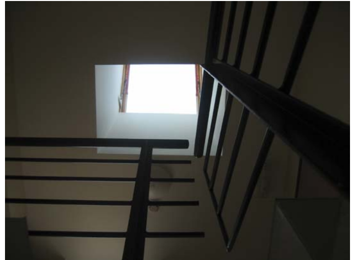
Smoke extraction openings at the top of the stairwell (source FEBELCEM)
