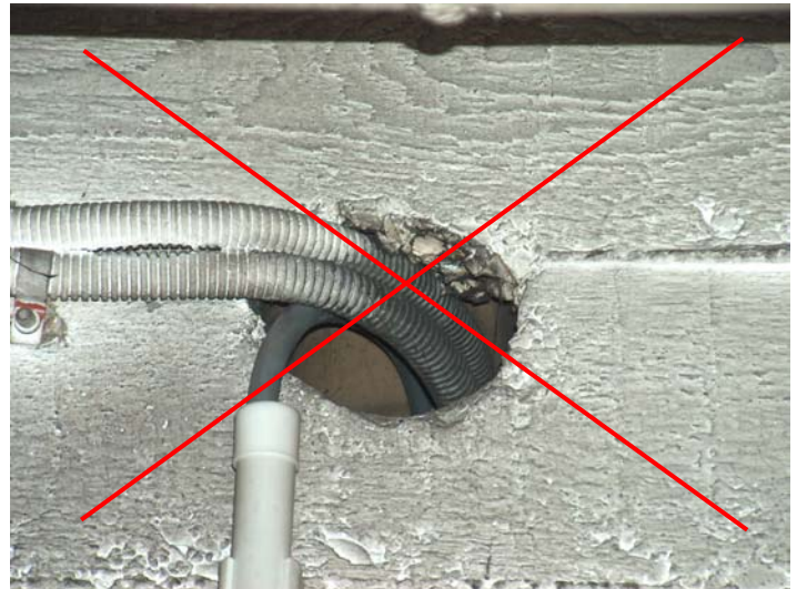
Avoid! An opening in an EI wall for passing electric cables through and which has not been re-pointed (source [8])
