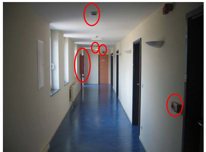
This corridor contains a large number of elements of active protection: alerting unit, hose reel, signalling panel, smoke detector, emergency lighting (source: FEBELCEM)
