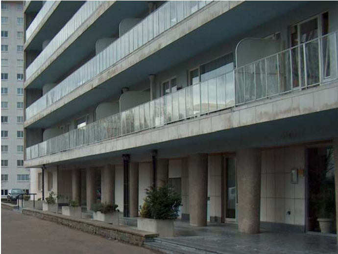
Walkways running along the entire façade of the building (source [8]). These continuous balconies constitute escape routes for people.
