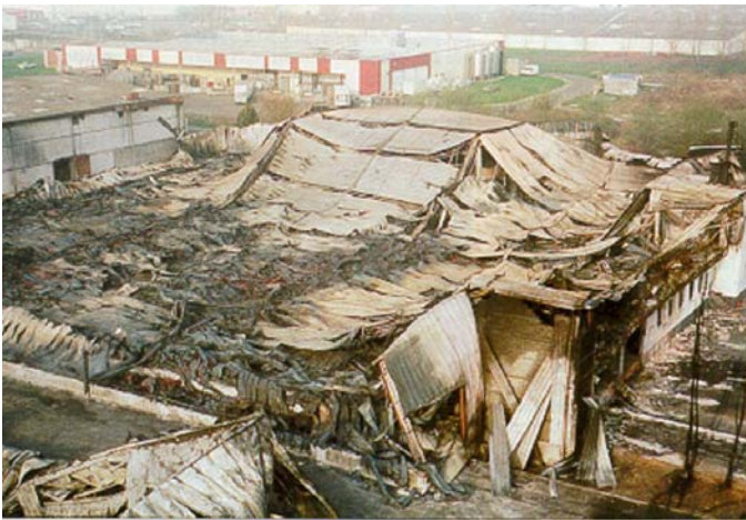
The risks of collapse are permanent and the risks of pollution are real (source CIMBETON)
