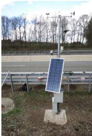
Image 6: Measuring station for measuring concrete temperatures, joint movements and climate data
